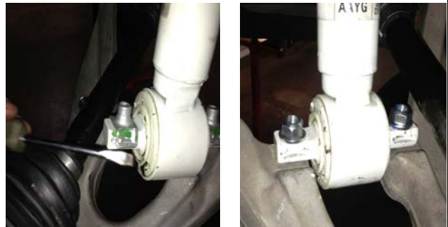
40. Remove the factory clips, attach the lower strut mount with new shorter hardware.
