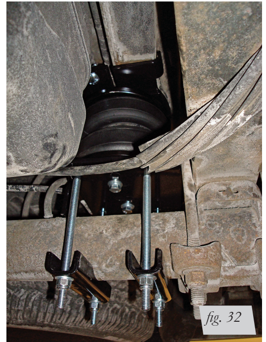
Left side (driver): front view of installation.
