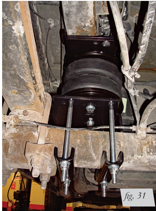
Left side (driver): rear view of installation.
