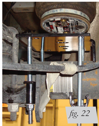
Right side (passenger) view towards front of finished installation torqued to 10ftlbs.
